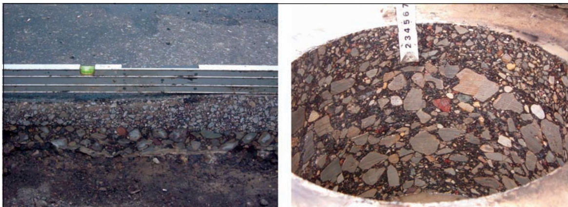
Fig 2. Borings made in the pavement structural layer and surfacing (structural layer of pavement: recycled mix ( h = 2 \times 10 cm) 50 % additive material, cold mix emulsion AEB-16 h = 4 cm)
