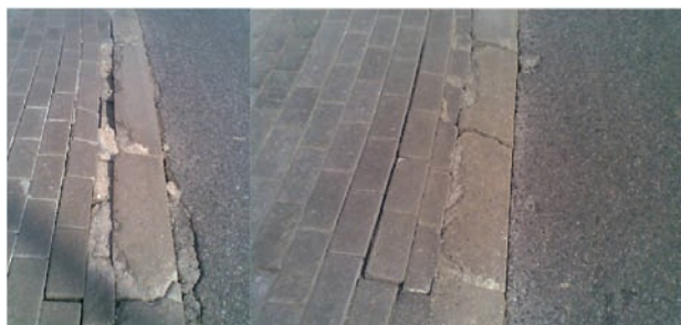
Fig. 12. Characteristic damages of road kerbs
