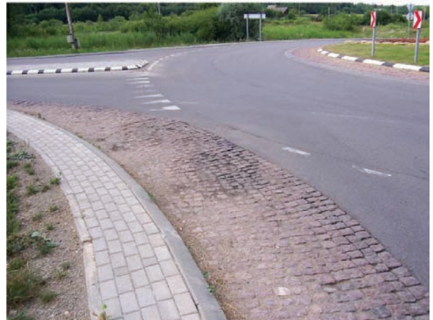
Fig. 11. The damaged block pavement on the widened carriageway
